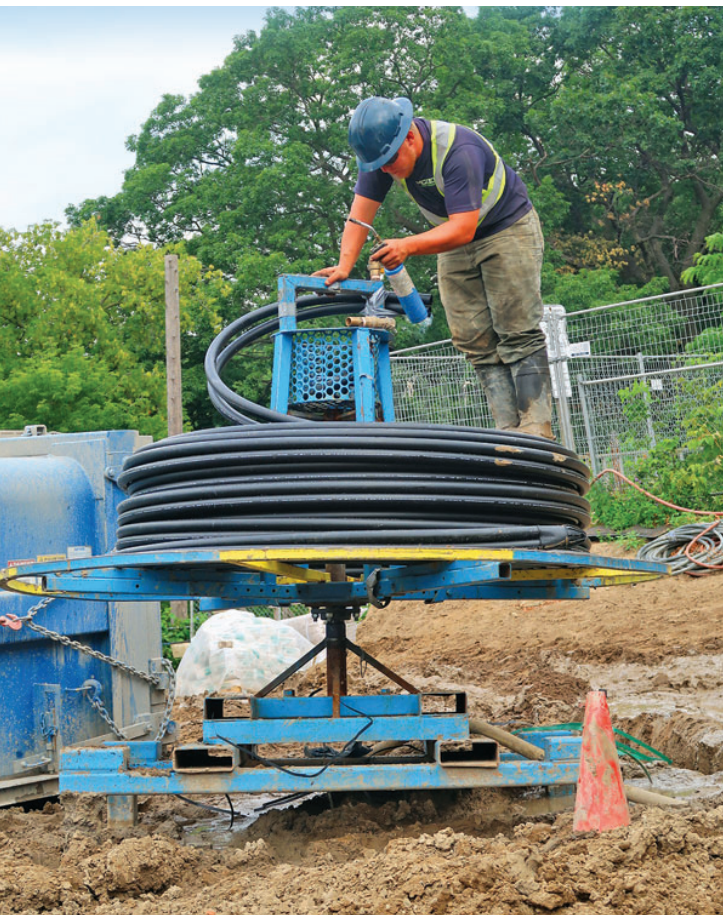
A worker prepares geothermal tubing as it is fed into the boreholes at Demirov's building.
