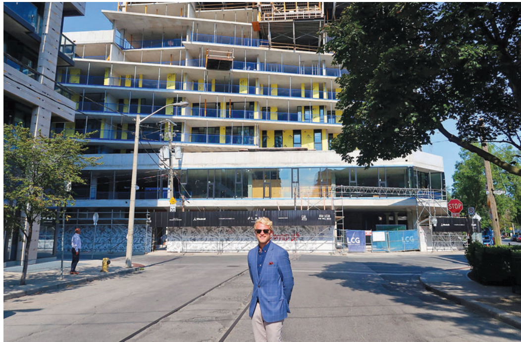
Diverso Energy’s Connor Stewart in front of The Plant, a large project featuring geothermal in Toronto’s Liberty Village.
