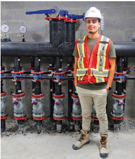
The Plant project coordinator Patrick Amorim displays the manifold for the geothermal system.
